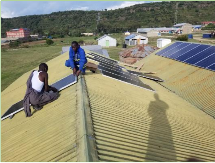
Borehole solar panels and the inverter at the borehole pump room
