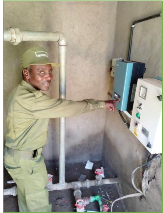
Staff member Lorot Ajiot in the borehole room ready to pump water
