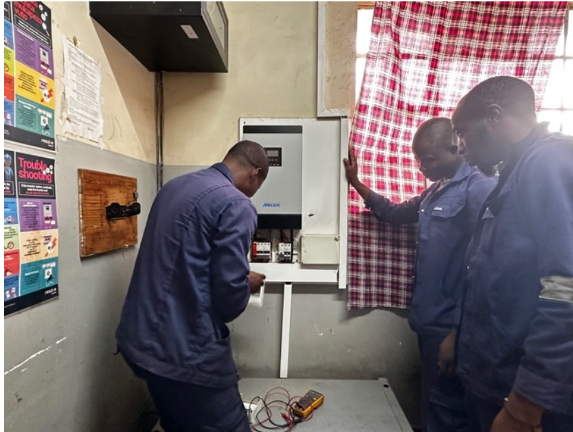
Solar technicians from Hi Tech inspecting the old and dysfunctional solar system.
