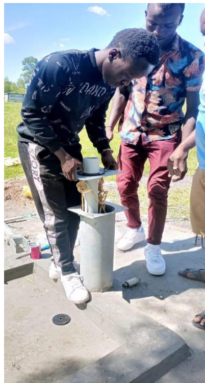
Pump installation at the well
