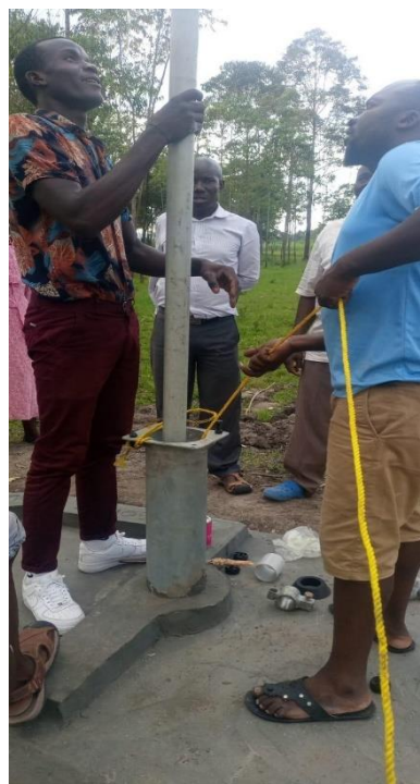
Pump installation at the well
